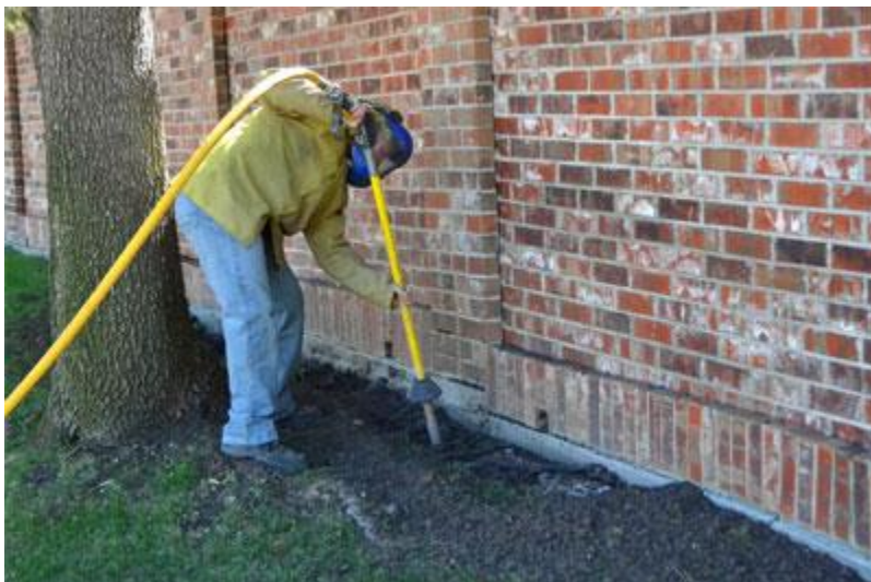
Pneumatic digging allows trenching through a tree's critical root zone without severing vital roots. Photo by Bill Seaman
